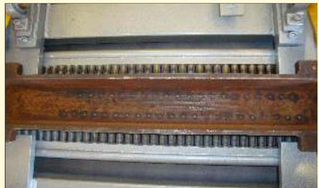
Gas burner and safety valve
